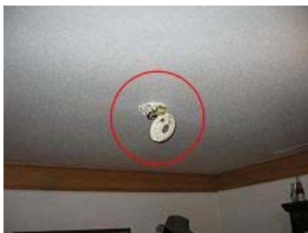
Photo 3 Smoke detector in the basement
